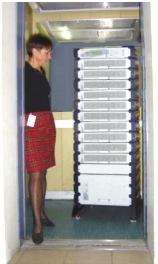
Figure 2: 100 kVA – Small enough to fit in a 4-passenger elevator
